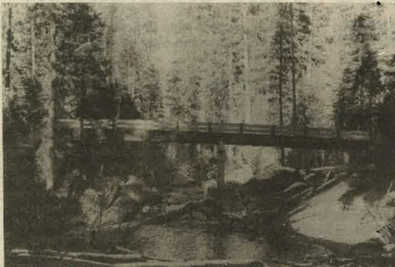
One of the bridges built in Caples Creek Roadless Area. Detail (below) shows that it was over-engineered. Photos by Craig Thomas
