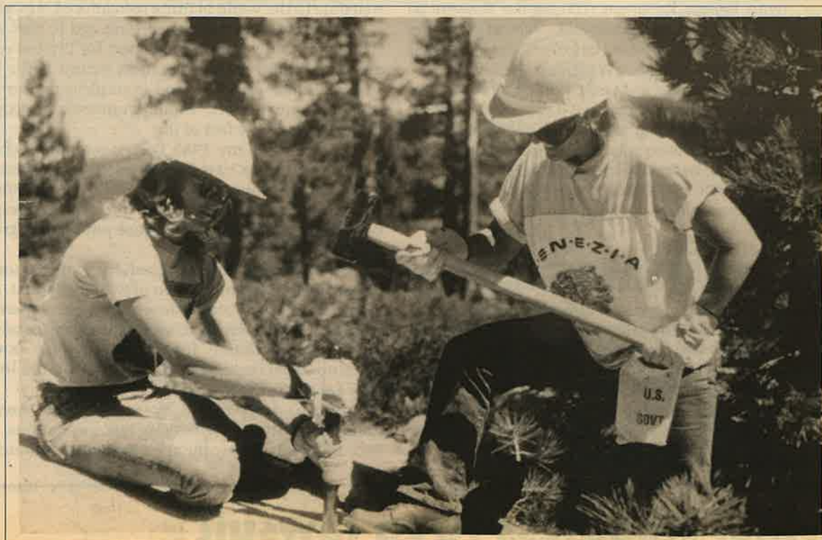
Trailshots trainees Karen Whitson and Mary McMillan use single jack drills to split rock while constructing the new Post Peak Pass trail. U.S. Forest Service photo
