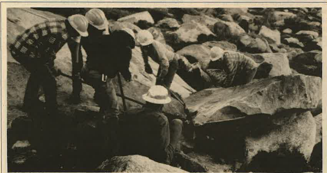
Boulders weighing up to 3 tons were moved during work on the Post Peak Pass Trail re-route; a total of over 180 tons of material were moved by hand over the course of the 1989 summer. U.S. F.S. photo
